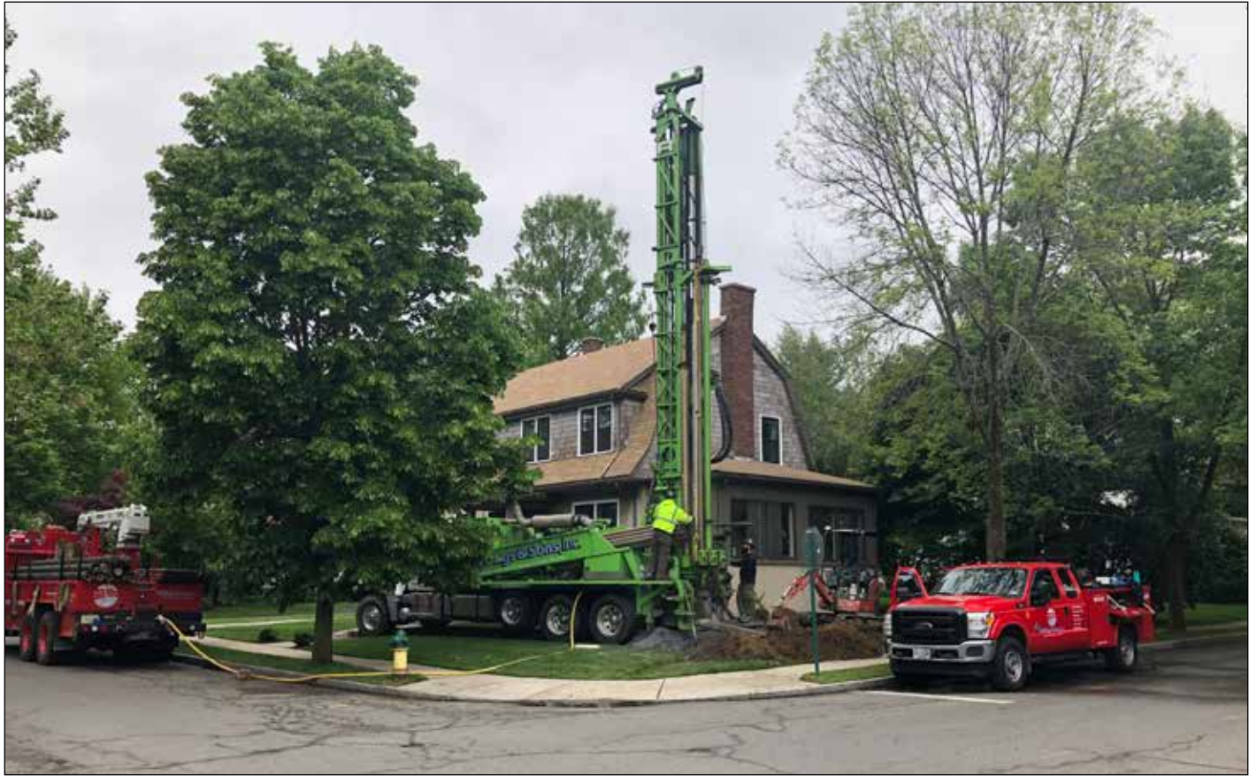
Drilling for a ground source heat pump at Katherine Oates' house, Belmont.
