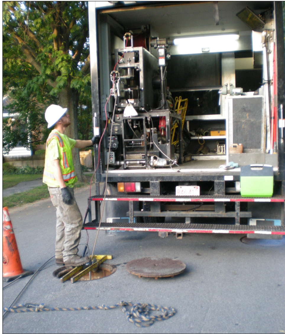
Figure 2. Crew member Chris Gouveia leads two camera cables into a manhole on Hoitt Road from the National Water Main Cleaning Company camera truck. Inside the truck, the crew foreman runs the mother camera.
