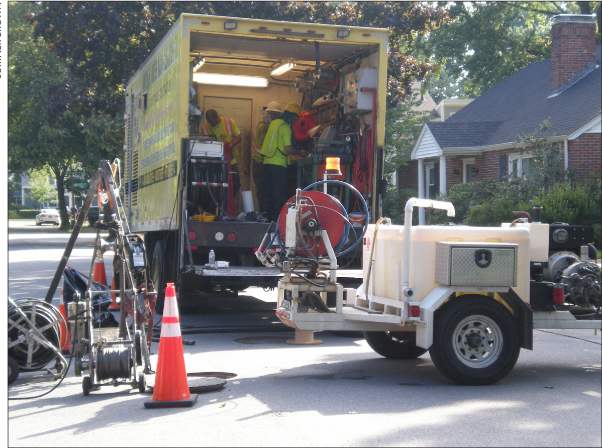
Figure 3. The lining truck carries the fabric and chemicals for the liner, as well as the steam curing equipment. The water trailer in front is for cleaning the lateral.
