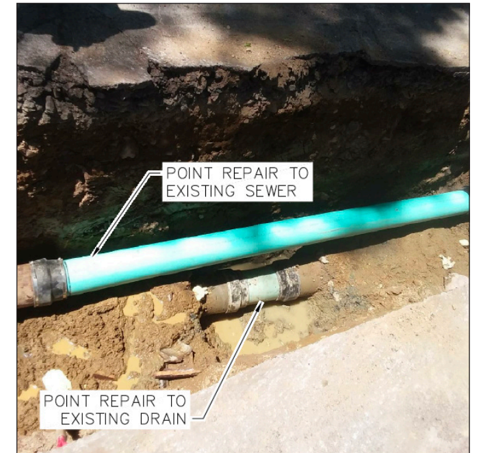
The sewer pipe is located above the storm drain in this repair under Homer Road.
