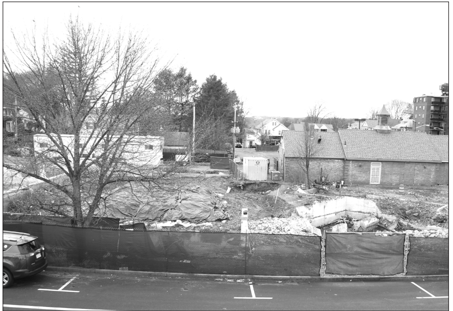
A partial view of the site from Common Street. The side of the Starbucks building, formerly Friendly's, is at right.
